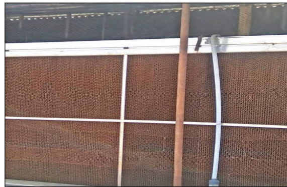
House with cooling pads
